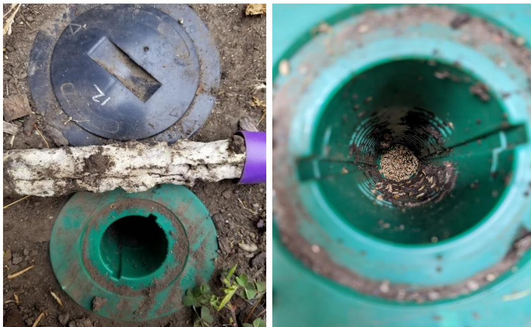
Figure 1. Sentricon Always Active bait tube damaged by termites (left) and associated bait station containing termites (right) approximately six months after installation at Berkeley site.
