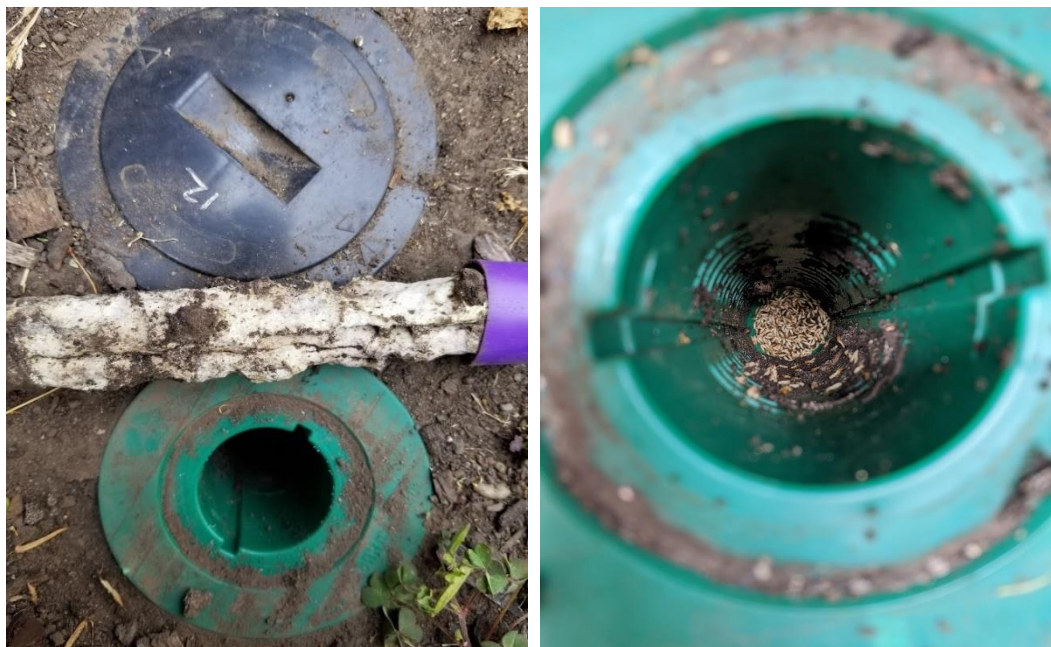
Figure 1. Sentricon Always Active bait tube damaged by termites (left) and associated bait station containing termites (right) approximately six months after installation at Berkeley site.
